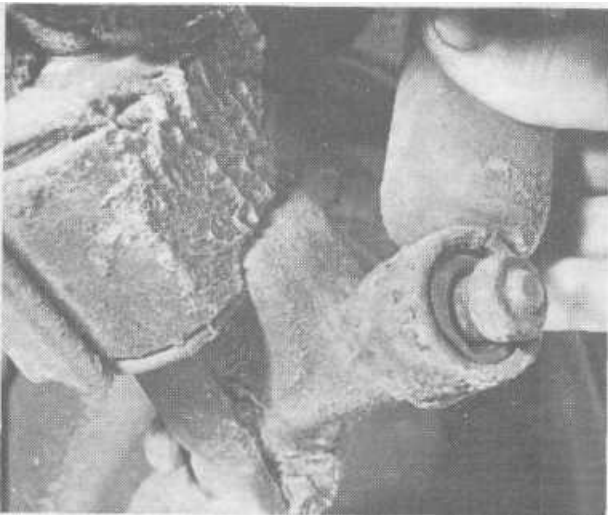
8.3 Inspect the shock absorber bushes. These need renewal
